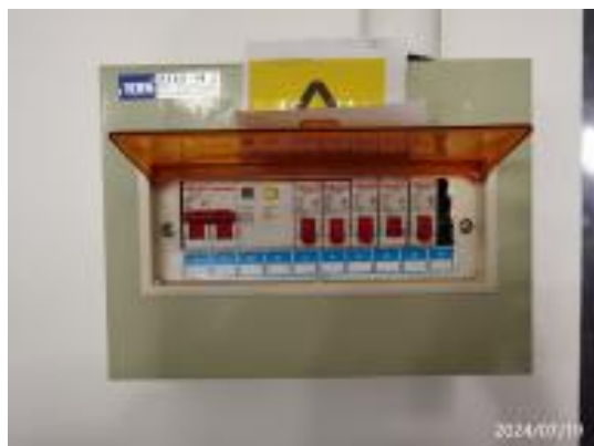
11. Electrical panel with cover.jpg
